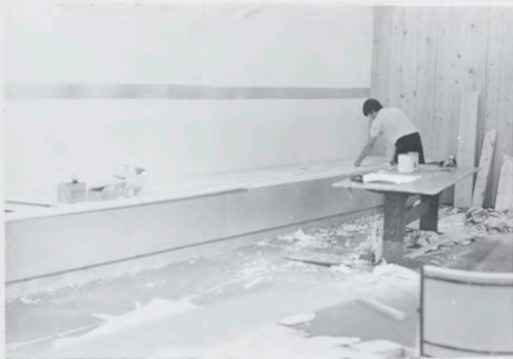
John measures up the area that the overshoot coverlets will go up in.
